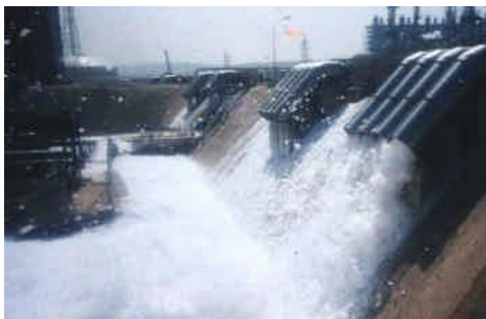
Angus Fire has designed many LNG fire protection systems worldwide
