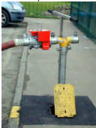
Hydrant test in progress showing typical equipment
